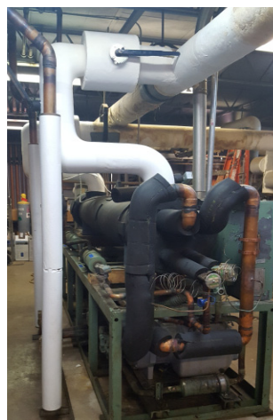
New Chiller Barrell
